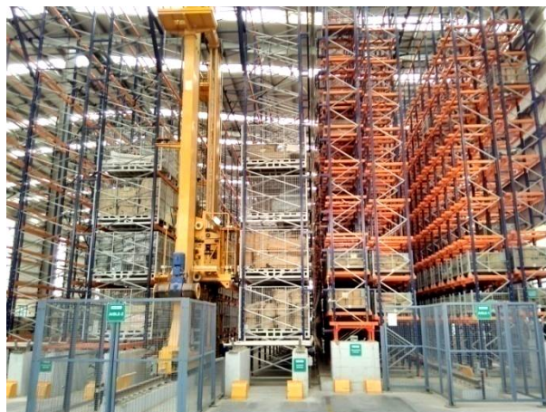
Automatic Storage and Retrieval System (ASRS)
