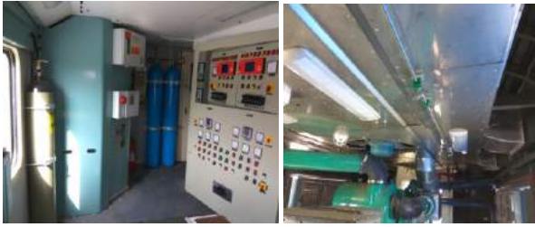
Automatic Fire Suppression System
