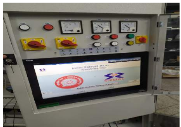
Smart Switch Board Cabinet
